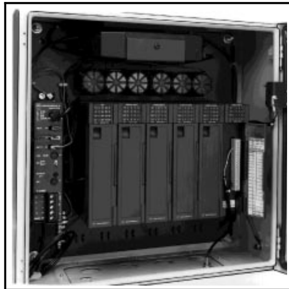
Figure 2. The MOSCAD RTU
